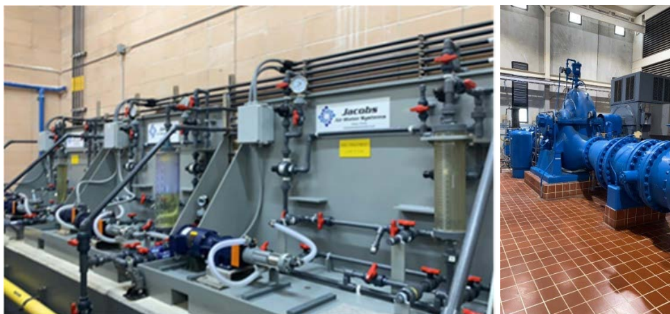
Figure 4-10: Cypress Creek Sodium Hypochlorite Feed Pumps and Finished Water Pump
