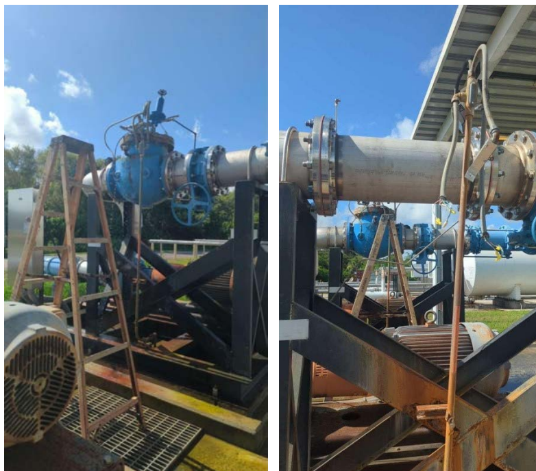
Figure 4-15: Alkalinity Adjustment Facility Carrier Pumps
