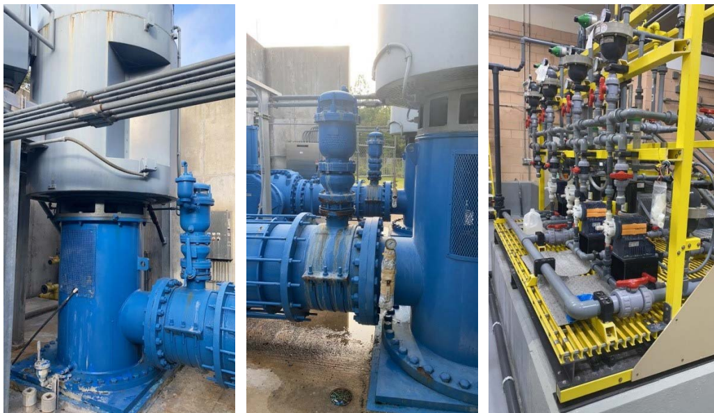
Figure 4-11: Morris Bridge WTP Finished Water Pumps and Chemical Feed Systems
