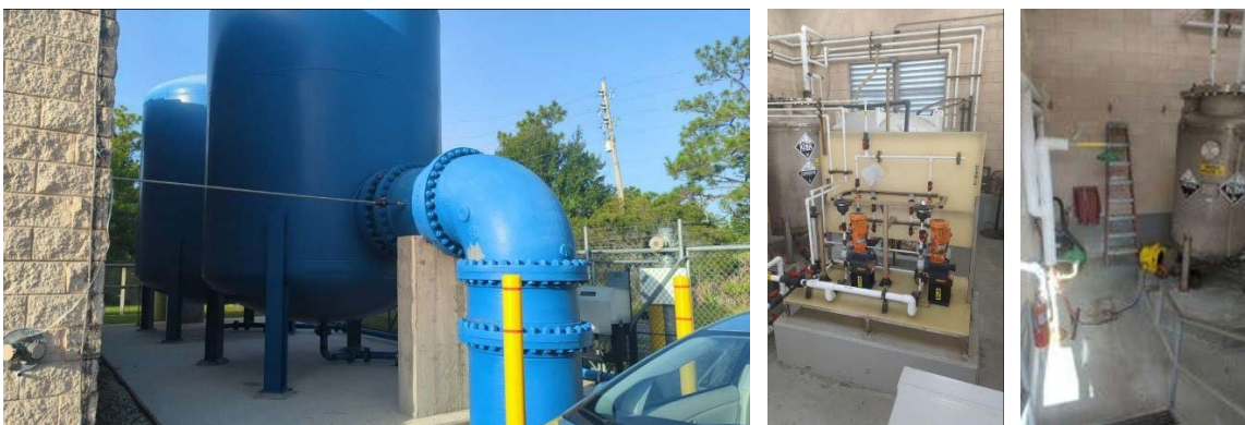
Figure 4-13: South Pasco WTP Chlorine Contact, Chemical Injection, Storage Tanks
