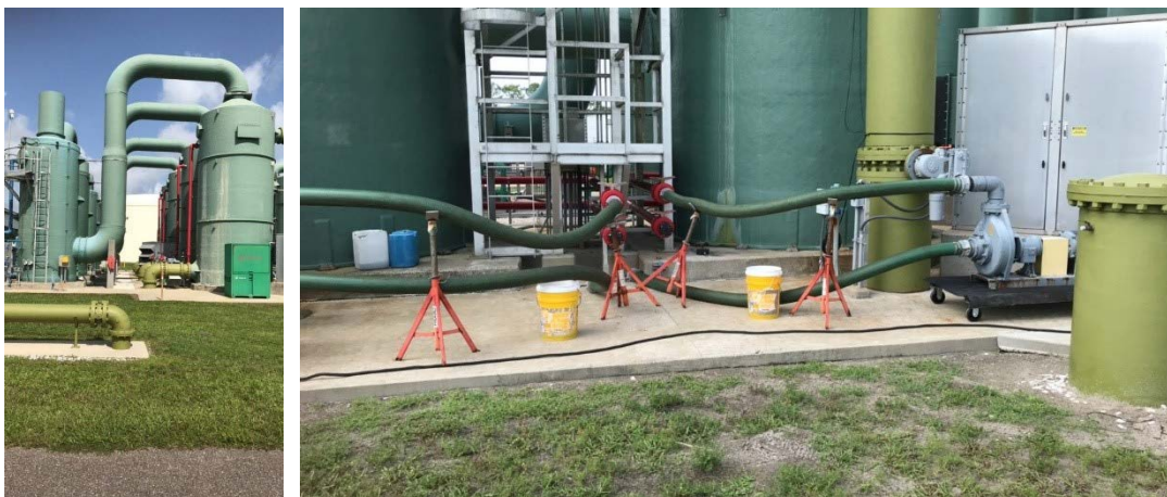
Figure 4-9: Keller Packed Tower Aerators and Temporary Pumping System
