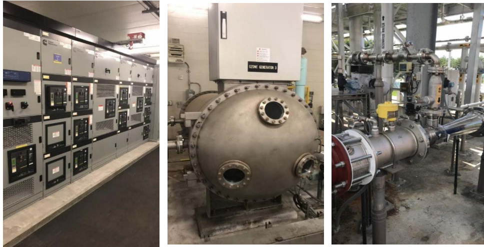
Figure 4-8: Lithia Hydrogen Sulfide Removal Facility Electrical Room, Ozone Generator, and Ozone Injection
