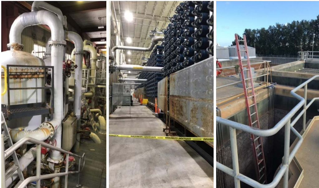
Figure 4-16: Tampa Bay Water Desalination Plant Diatomaceous Earth Filters, Reverse Osmosis Process, Lamella Basin
